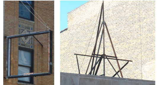
Sample chain and A-frame signage
