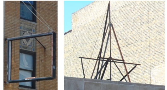
Sample chain and A-frame signage
